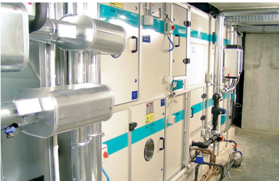
Adiabatic air conditioner using rainwater.
