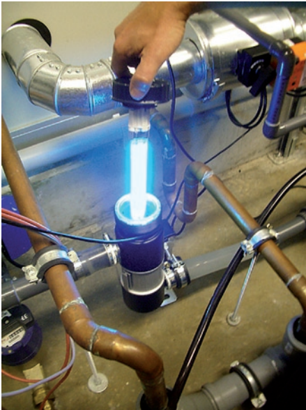
UV waste water disinfection
