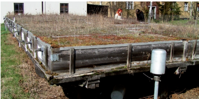
Measurement of evaporation and runoff from different types of extensively greened roofs (5 cm and 12 cm of growing media, s. Fig. p. 12)
