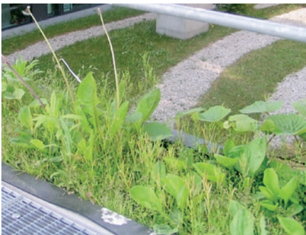
Weeds have become established in these rather inaccessible planters and are competing strongly with climbing plants and
